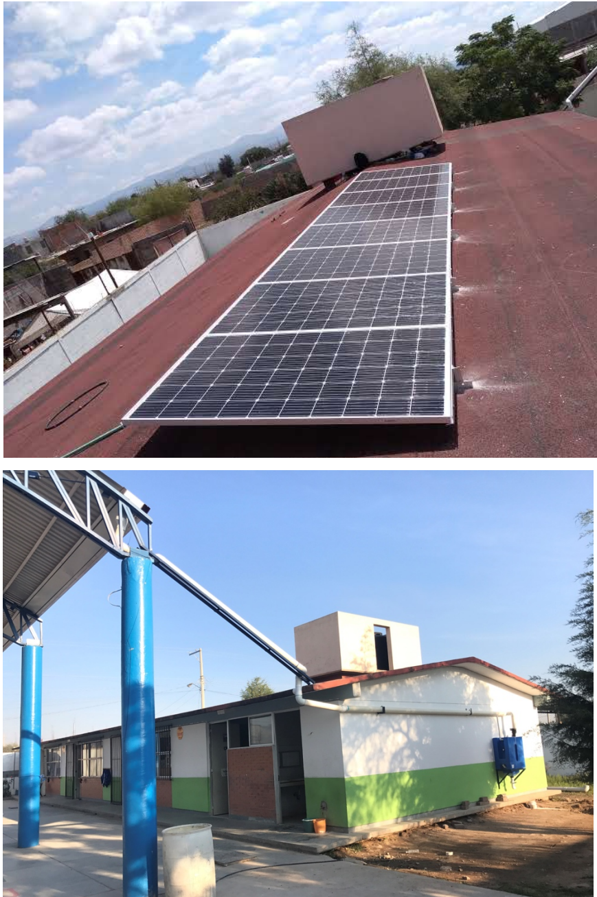
Figure 19. Ecotechnologies on the Pilot School. Project Database.
