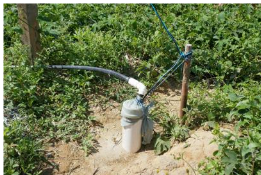
(a) Artisan water well is deeper and has a PVC tube with a small diameter. The water is extracted without a pump.
