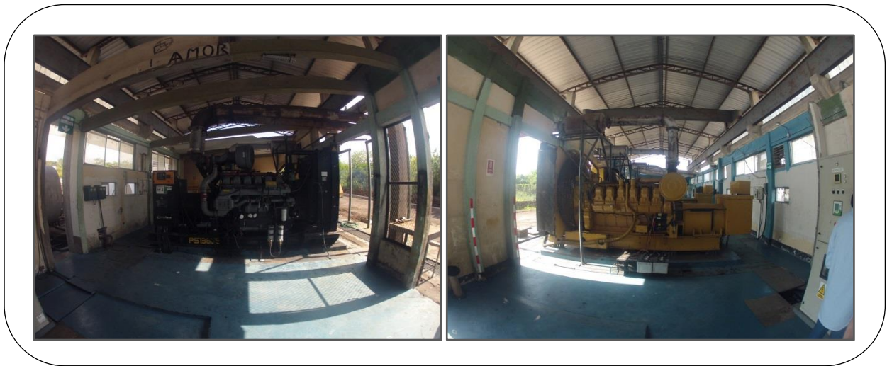
Figure 15: Diesel Generator in San Cristóbal
