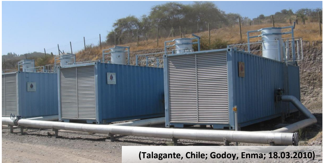
Figure 15. Horizontal flame torches
