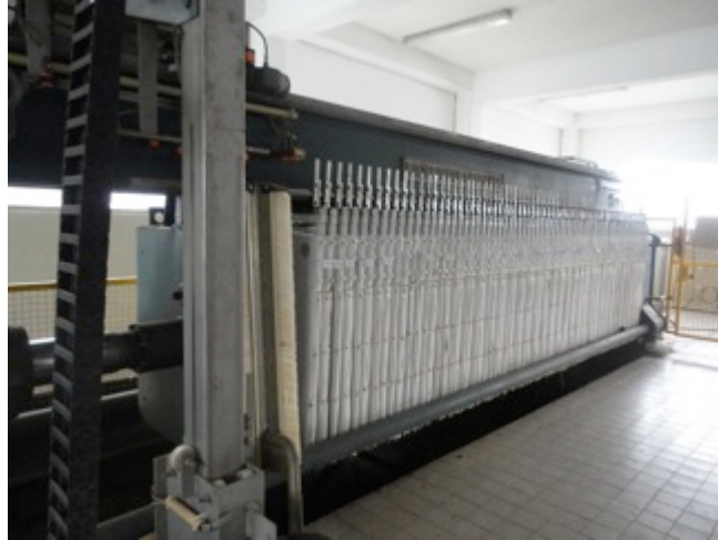
Figure 5. Filter Press Beningsfeld Wastewater Treatment Plant
