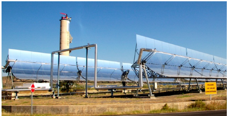
Picture 1: Parabolic Trough System: DISS Source: (Ciemat, 2010)
