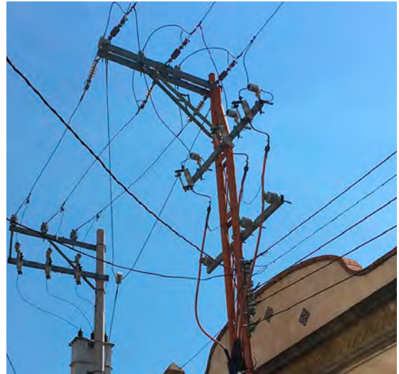
Blue sky with cables | Cielo azul con cables
