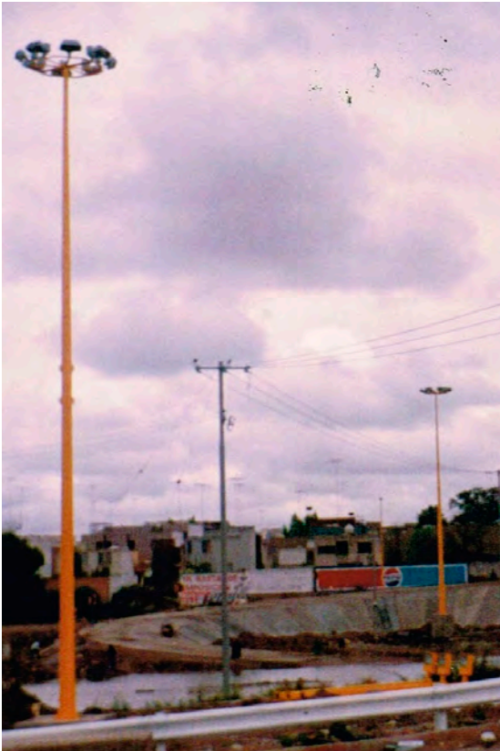
Streetlight installed | Alumbrado instalado
