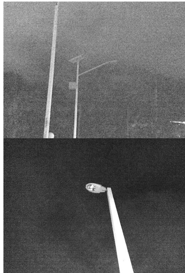
Figure 25 - Condition of the decentralized solar public lighting system in SLP. Source: Own elaboration.
